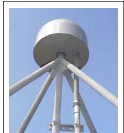
Figure 7. SCIGN station NOPK - 'as built'
