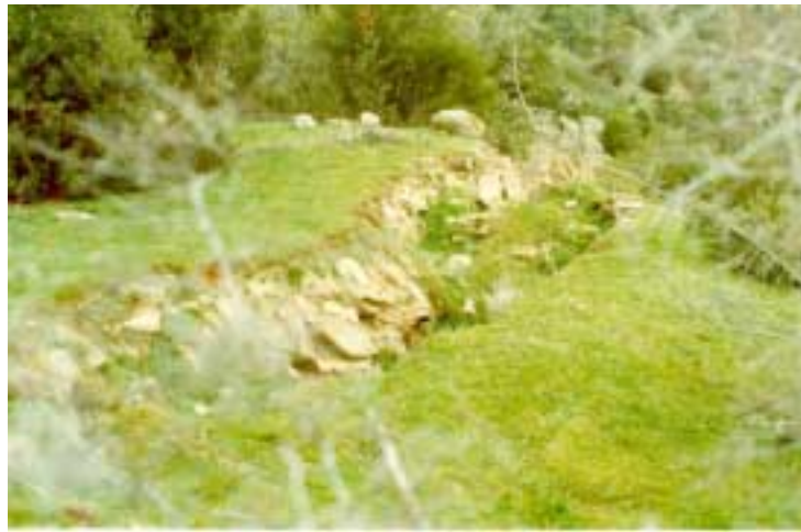
Figure 3: A ground rupture of the ‘Beta’ landslide.
