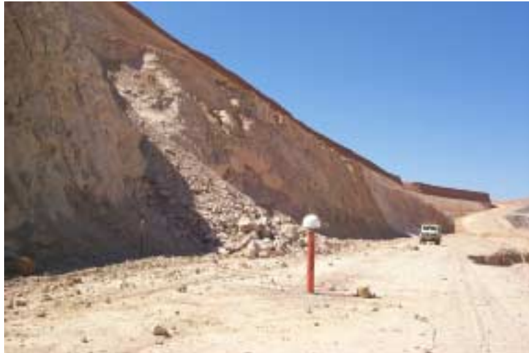
Figure No. 4: Deformation station 3 situated near to the mine wall and below top excavation level
