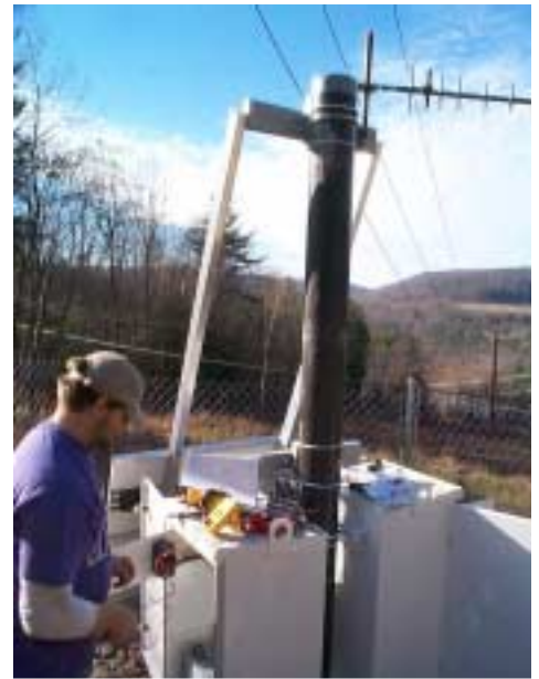
Photo 2. Installation of battery array and GPS sensor at Station REM1.
