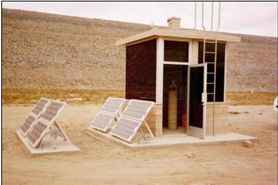
Figure 6. RTS observation shelter.
